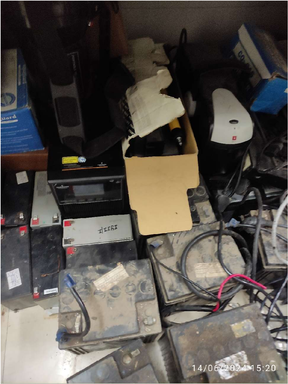
UPS 3 KVA Accutech (3 Qty at NIRRCH)
